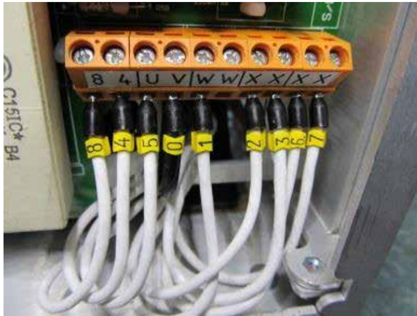
The picture shows 240VAC arrangement.
